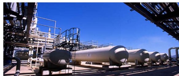
Compressed Air Supply System (3,5kg/s)
