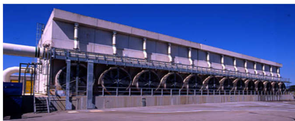
Tower Water Supply System (11700 m 3 /h)
