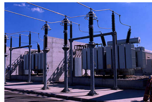
Electrical Energy Supply System (90MVA)
